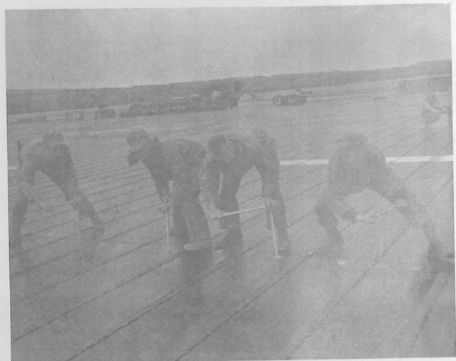
Marines are here shown tightening sections of the M9M1 extruded aluminum planking used to surface SATS runways. It is watertight, flexible at the joints and can take the aircraft wheel and tail hook impact loads.
